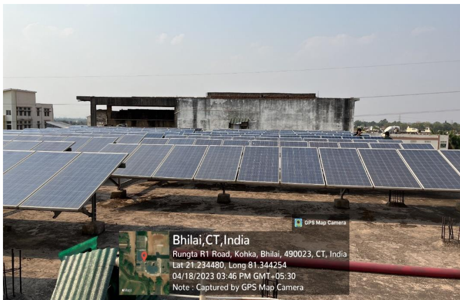
Solar panel of 100 kW capacity
