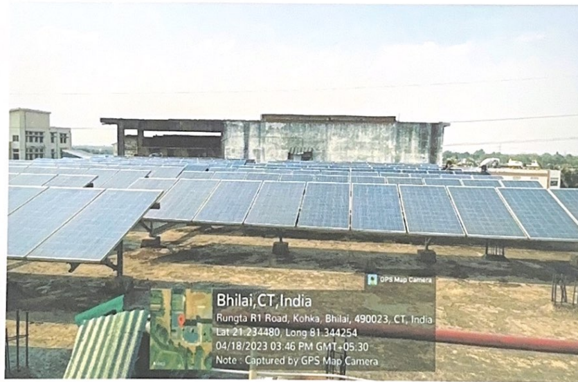
Solar panel of 100 kW capacity
