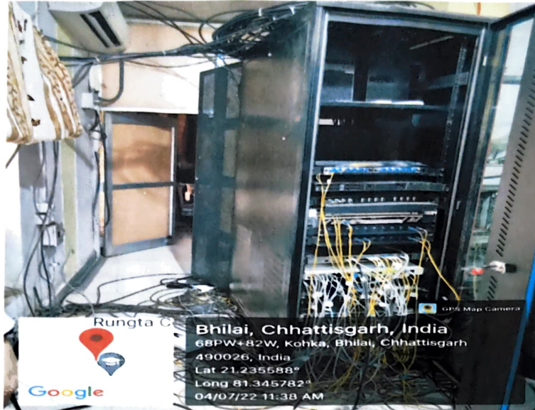
Pic: Server Room
