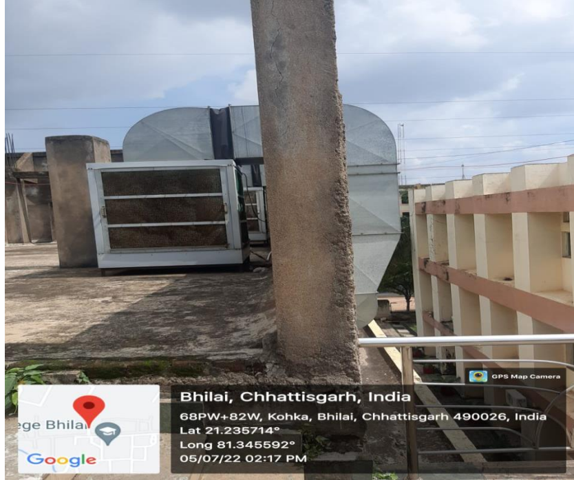
Pic: Centralized cooling system
