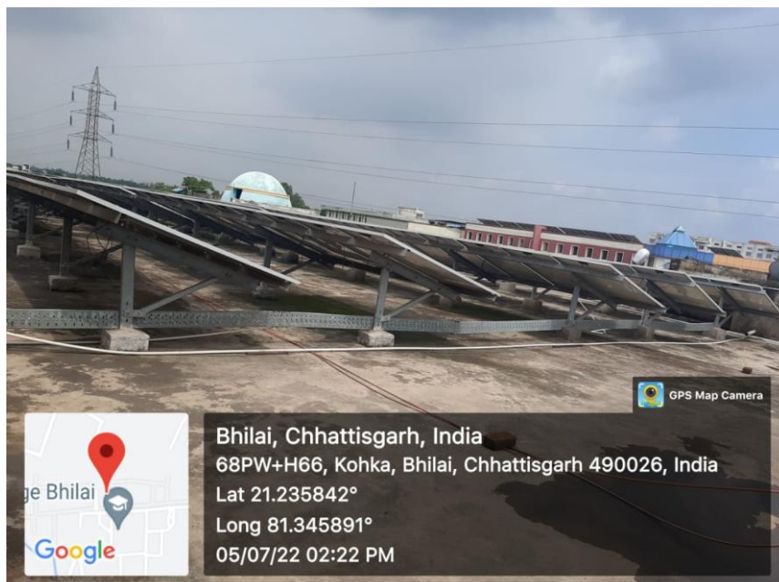
Pic: Solar Pannel
