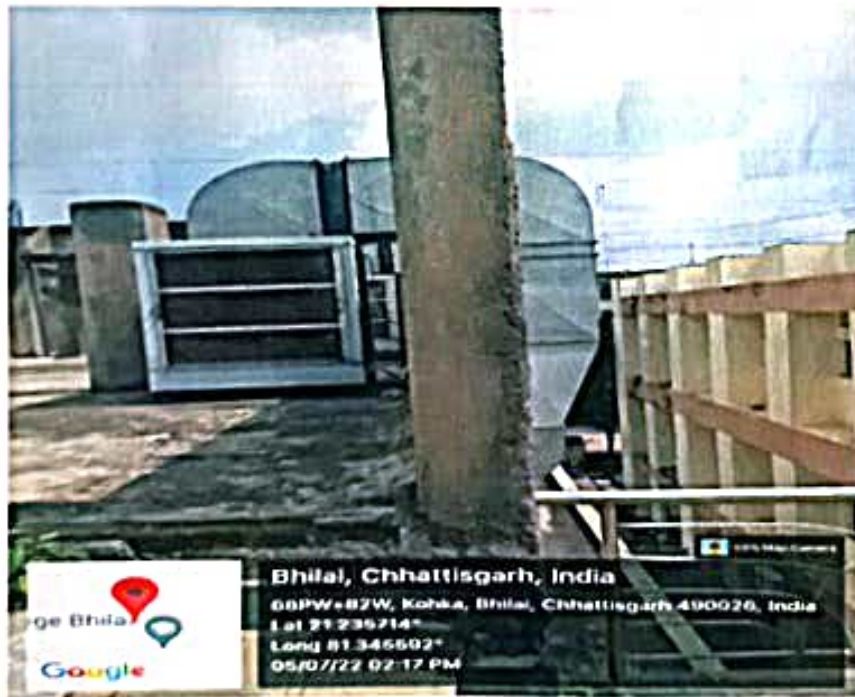
Pic: Centralized cooling system
