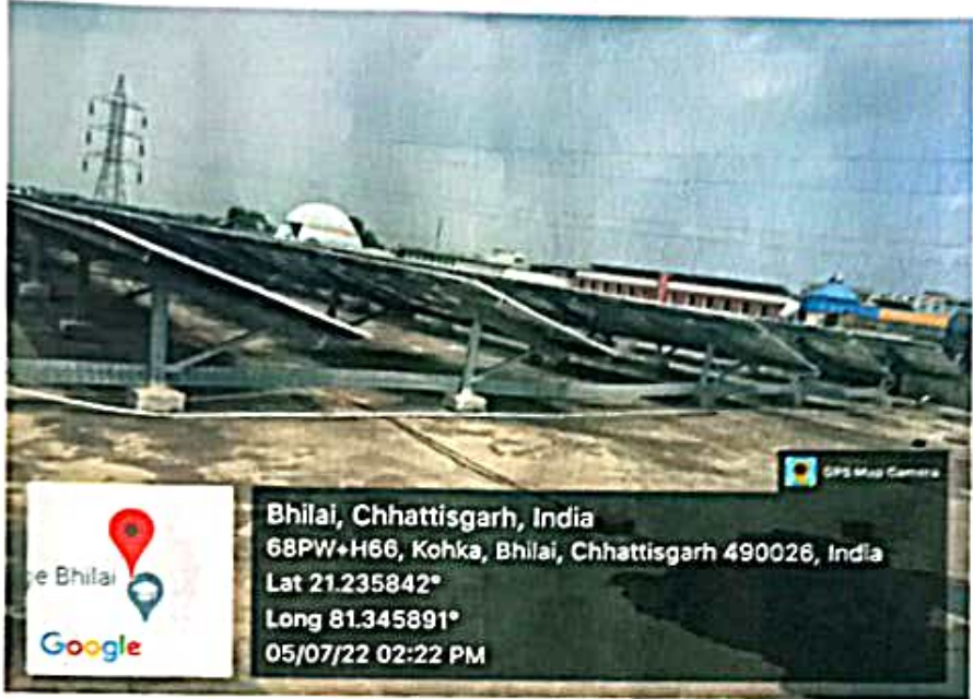
Pic: Solar Pannel
