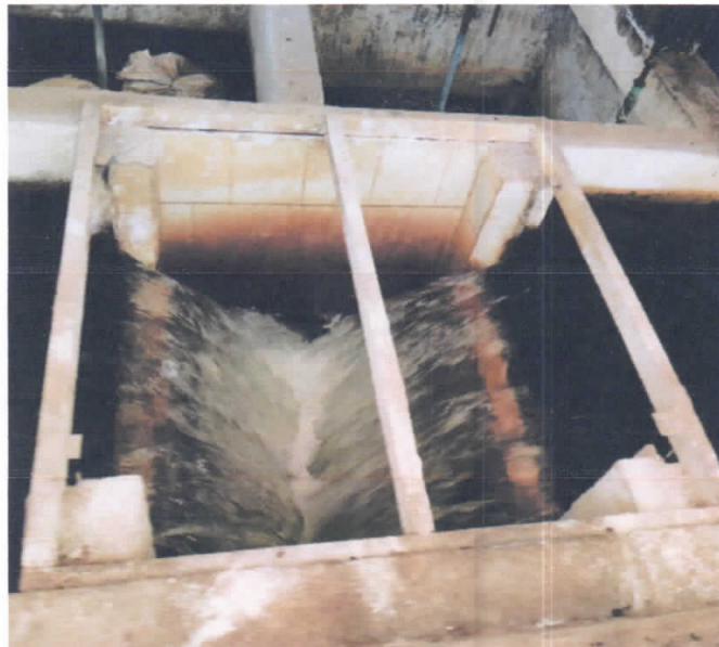
Disinfection of water
