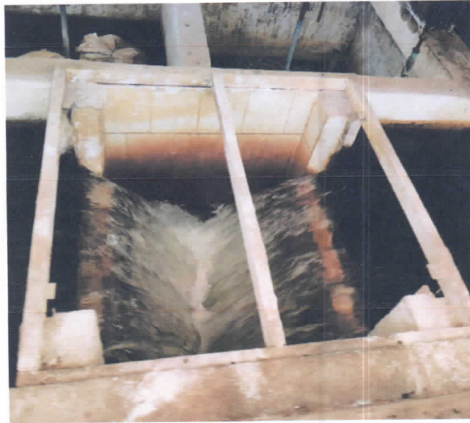
Disinfection of water
