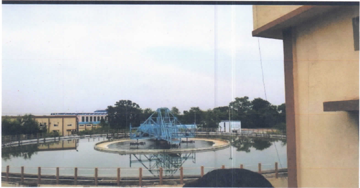
Picture of Water Treatment Plant
